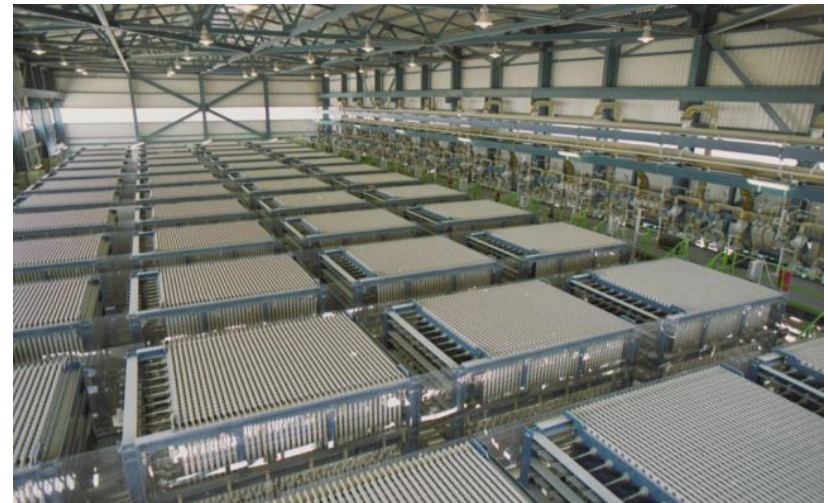
Chlor-alkali cell room – Uhde GmbH
